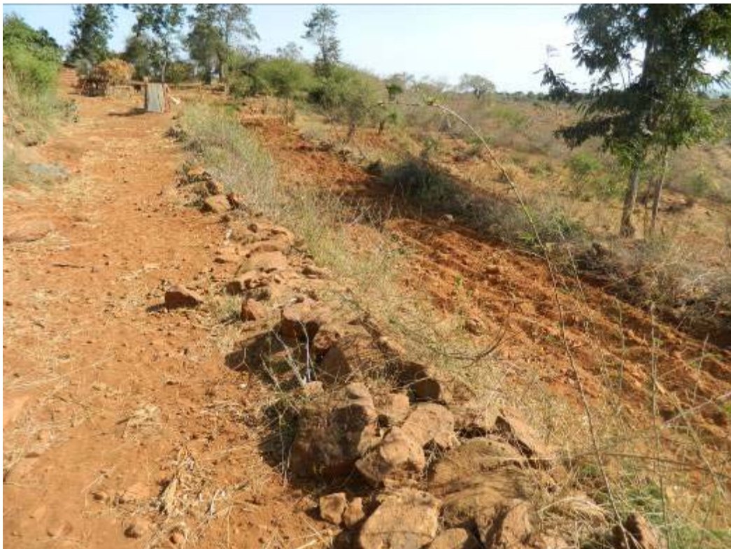
Stone berms for controlling runoff, partly vegetated, stabilizing the slope and terrace foot
