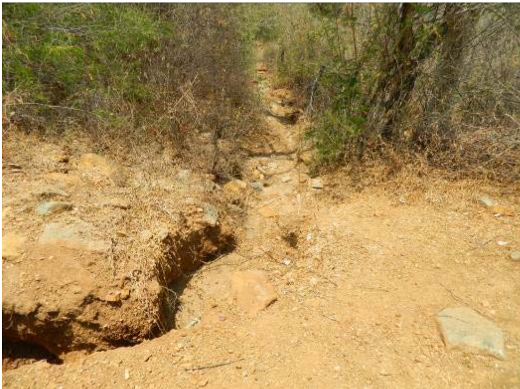
Water finds an unmanaged path away from the road causing erosion on downhill agricultural terraces
