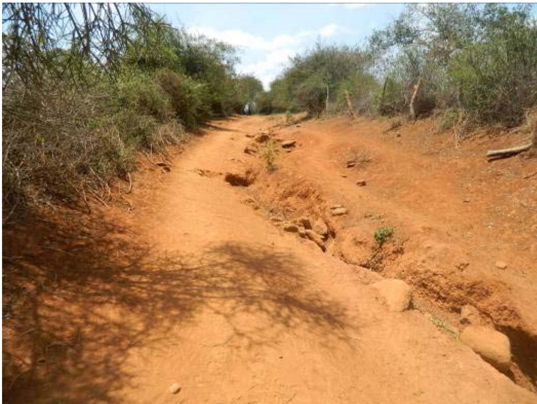
Erosion and forming of gully on access road 100m downhill from plateau
