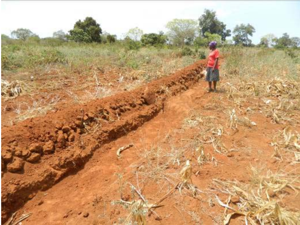
Newly established bench terrace (“Fanya juu terrace”), steep slopes will erode immediately with the first rainfall, seed and/or mulch to establish anchoring vegetation
