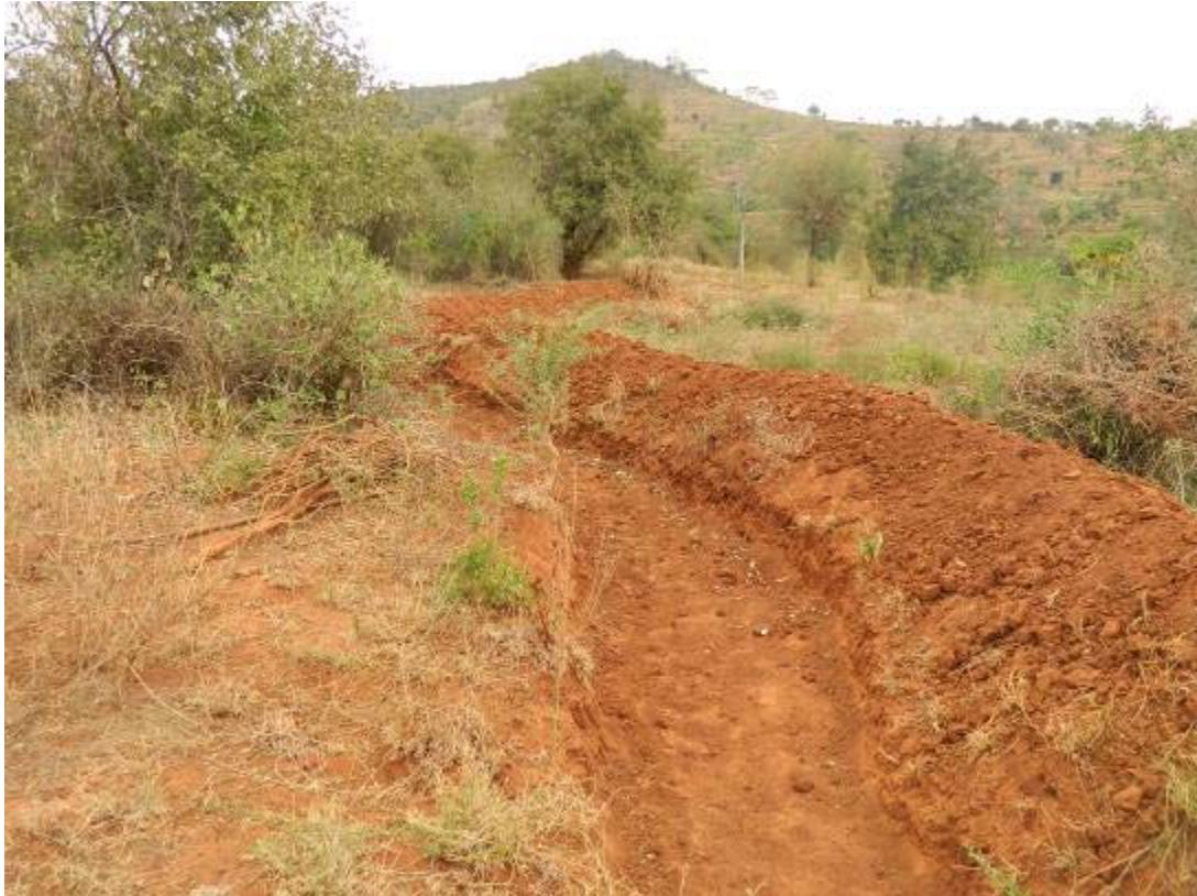
Hand dug swale for the avoidance of runoff and erosion, benefiting infiltration
