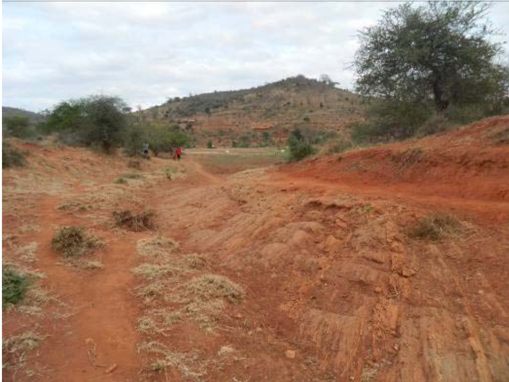
Spillway of Musosya earth dam, increased runoff starts to erode the dam, this has to be immediately repaired to avoid a total dam failure
