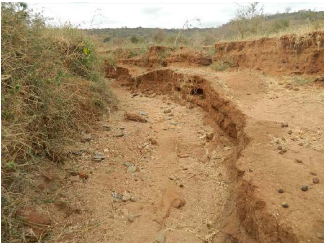
Gully development in two phases, sign of increase of runoff and eroding forces Secondary gully eroding the terraced land
